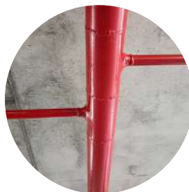
Joint fire extinguishing system pipes
