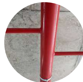
Jointless fire extinguishing system pipes
